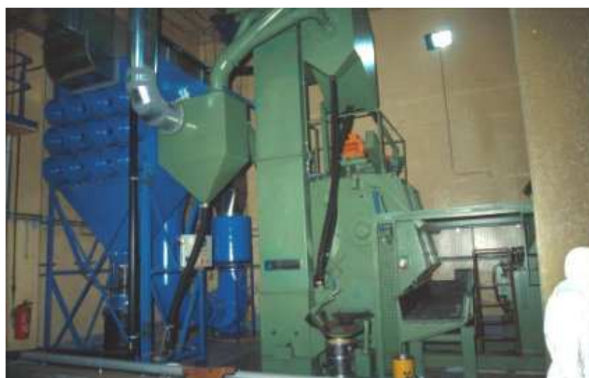
Figure 2. Operational view of the abrasive blasting installation
